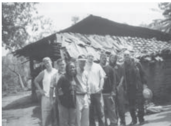
Stan Ingman and a group of workers on a field trip to fix a roof at a house in the mountains above Dos Aguas in Mexico.
